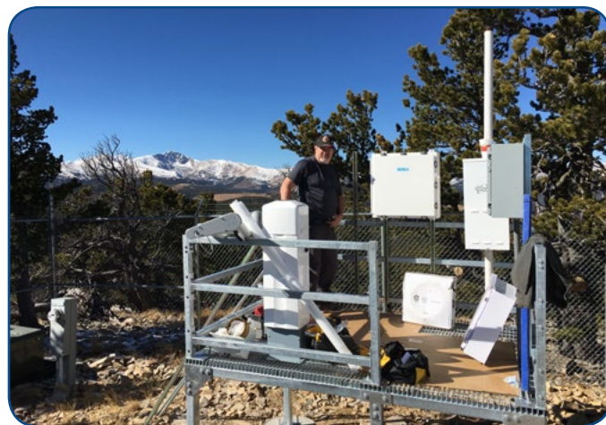
Governor's Office of Information Technology (OIT) Technician Curtis Nations performs the installation of the new Dakota Hill AWOS near Central City, Colorado. Photo Shahn Sederberg. VIDEO LINK: Colorado AWOS Maintenance.
